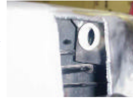
View of the bushing support from side.
